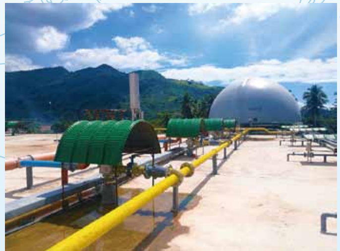
View from on top of the digester boxes: flare, pipeline and gas holder
