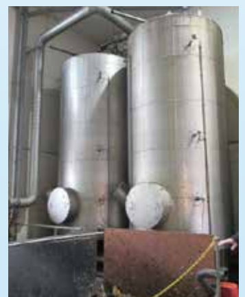
Commercial waste hygienisation vessel
