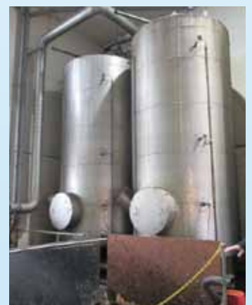
Commercial waste hygienisation vessel
